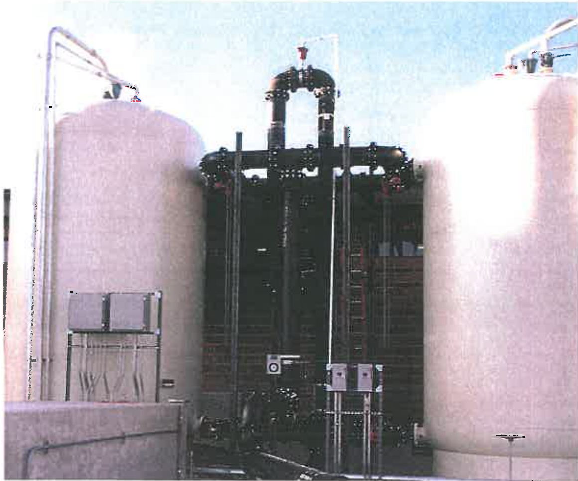
Figure 4-3 GAC Contactor Vessels (Courtesy Tonka Equipment Company )
